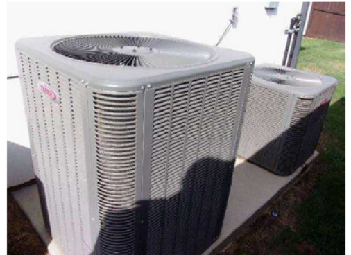
Condensing Units (typical)
